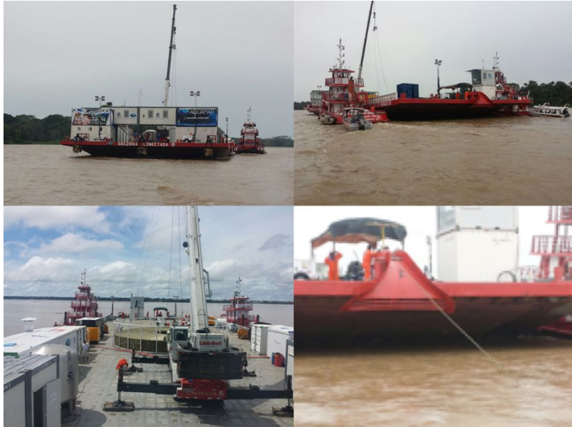
Fig. 19 Laying the pilot project cable from Coari to Tefé: Above: prow (L) and stern (R) of the barge. Below: the cable “tank” (L) and the paying out of the cable from the stern (R).
